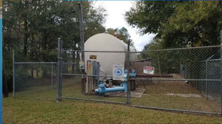
Water facility at The Meadows subdivision, just off Airport road south of planned residential area.
