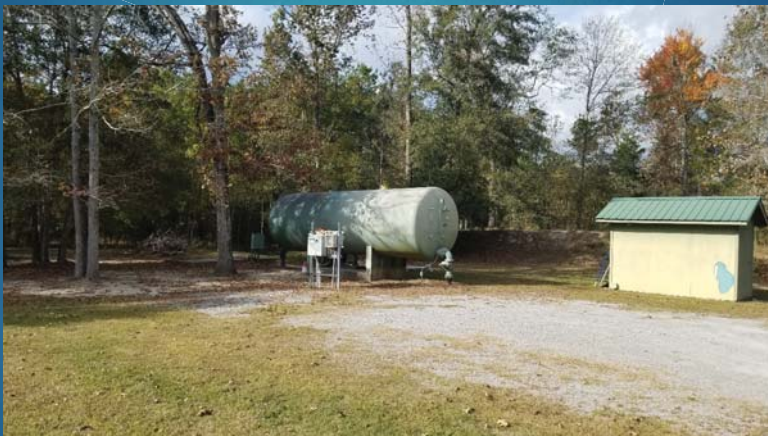
Water facility at Brier Lake subdivision, south of I-12 just west of Salmen Fritchie property.
