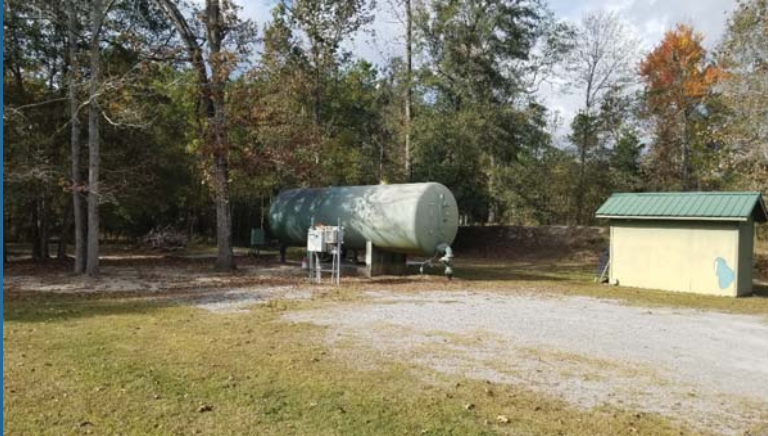
Water facility at Brier Lake subdivision, south of I-12 just west of Salmen Fritchie property.
