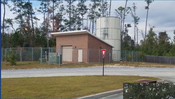
Water facility at Mayfield Elementary, south side of US 190 just across from Salmen Fritchie property.
