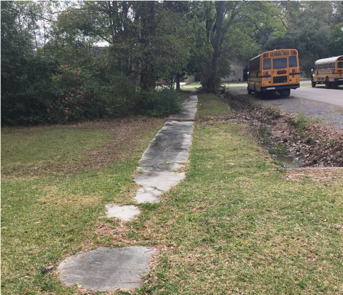
Figure 2.4: Poor Sidewalk Condition (W. 18 th Ave. facing east to S. Jefferson Ave.)
