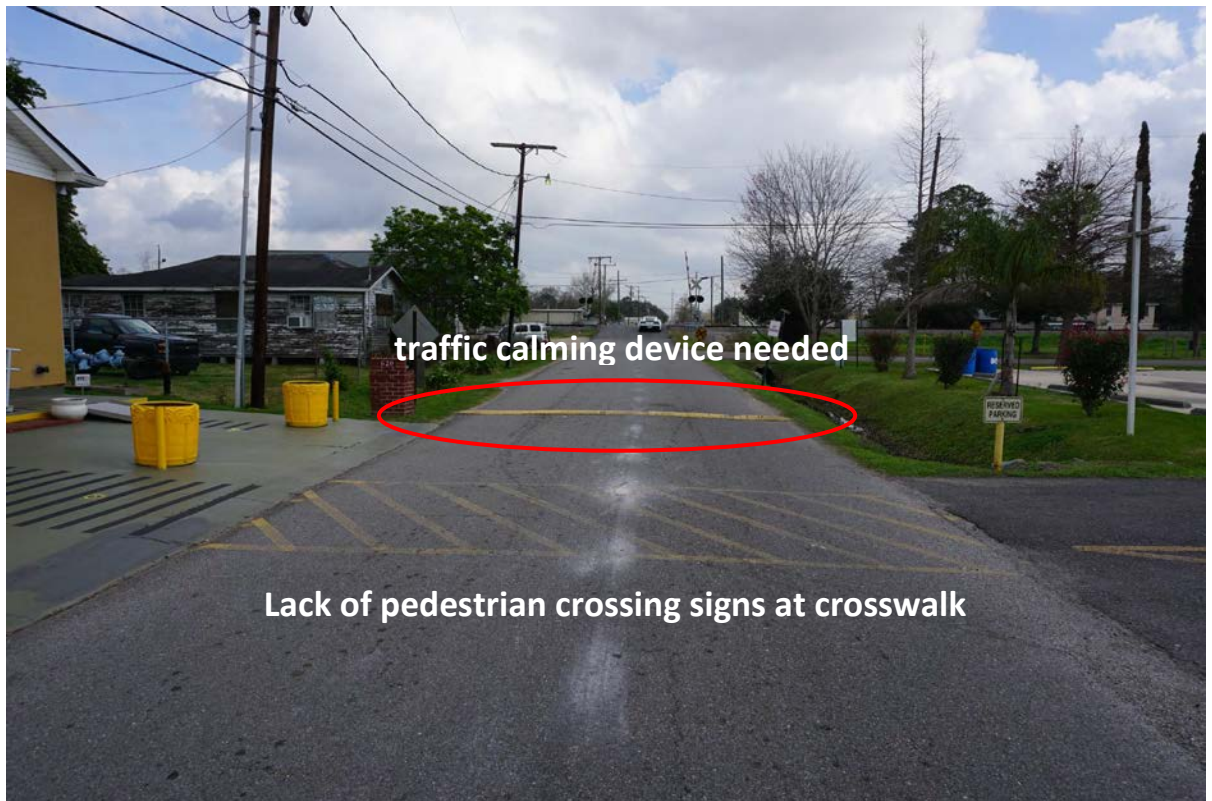
Image 25 – Cardinal St. - overhead utilities, large open drainage, and traffic calming devices Photo Credit: DDG 2/14/17
