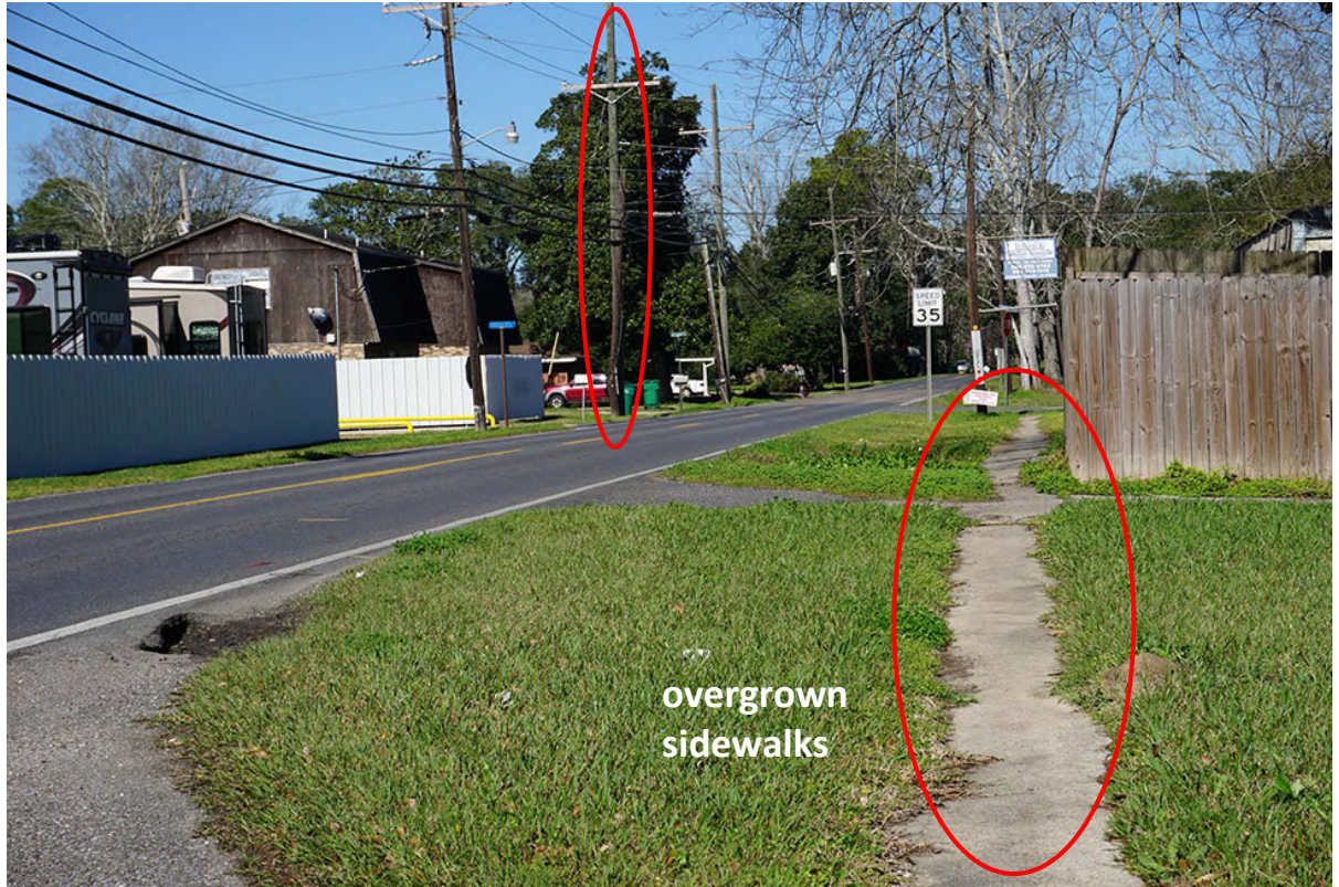
Image 36 – E. 5 th St. – overgrown and damaged sidewalks, overhead utilities, and driveway conflicts Photo Credit: DDG 2/14/17
