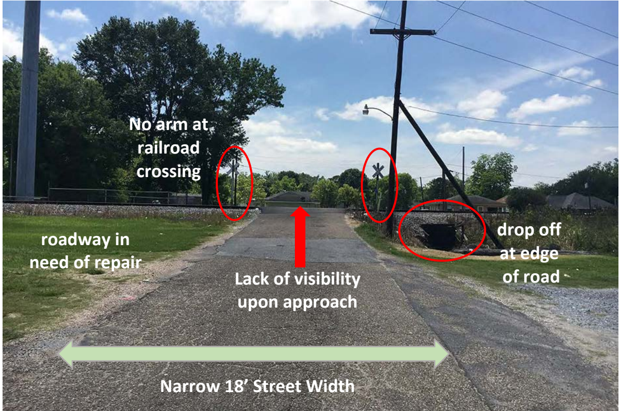
Image 18 – Spruce Street at Railroad - overhead utilities, narrow damaged street, steep grade at ditch Photo Credit: DDG 2/14/17
