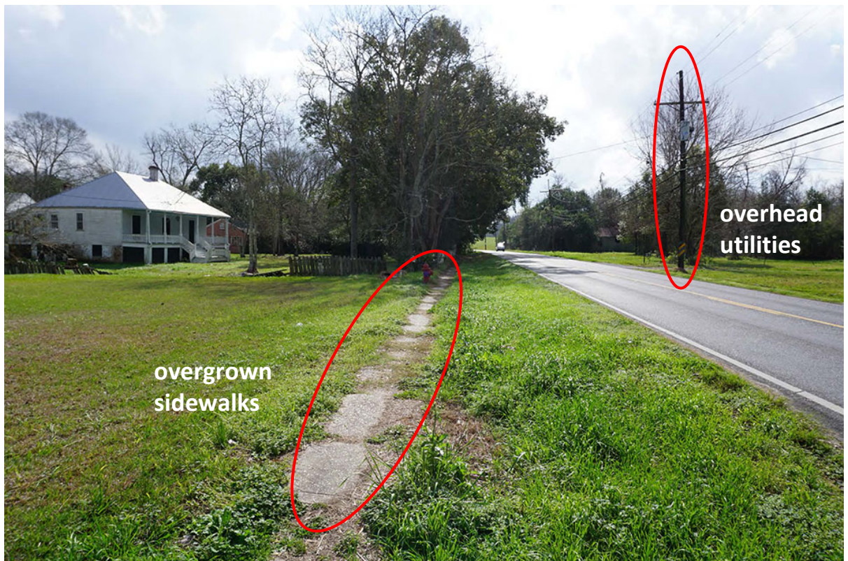
Image 37 – E. 5 th St. – overgrown and damaged sidewalks, overhead utilities Photo Credit: DDG 2/14/17
