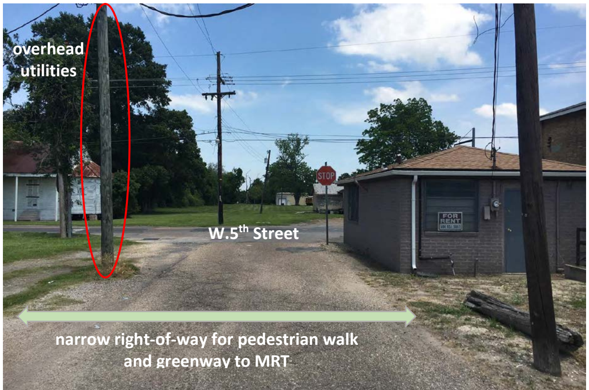
Image 17 – Spruce/5 th Street - overhead utilities, uncontrolled parking, pavement failing, narrow street Photo Credit: DDG 2/14/17
