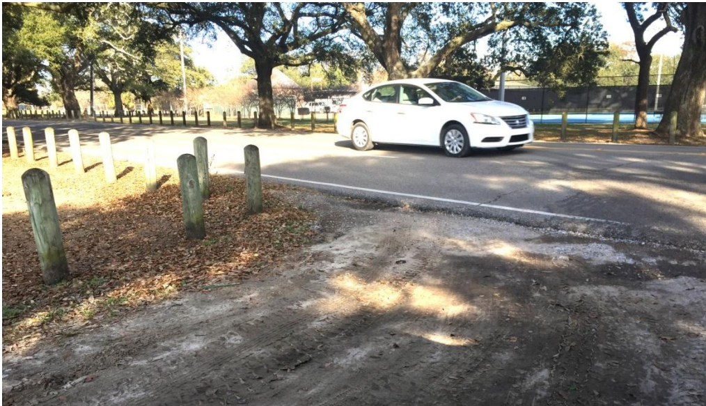
Photo 10: Parking area connection to Marconi Drive abrupt height change.
